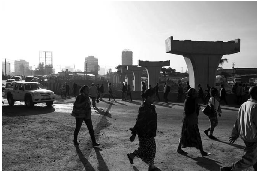
Figure 6b. Mexico Square: current situation during construction/demolition; view towards east. (Photo: A. Thorer, 21 May 2014)
