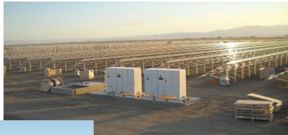
Solaron PV inverters, 500 kW, installed at a 35 MW PV plant, near Coalinga, CA
