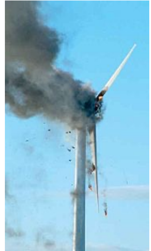
A turbine on fire after an oil leak
